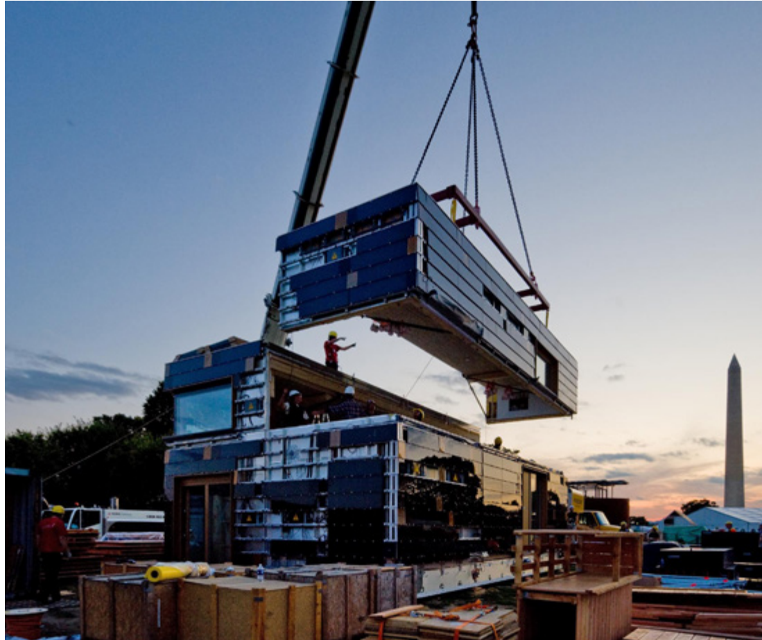
↘ [Construction Photos] Solar Decathlon Prototype, Team Germany / TU Darmstadt, 2009. Photos Thomas Ott 2009
